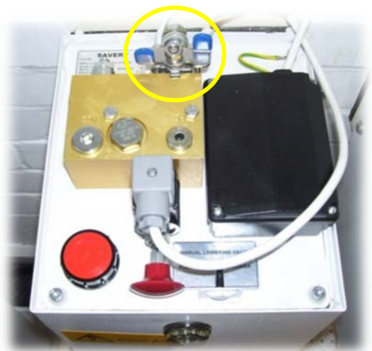
Fig 11.1 – Shut-off valve shown in ‘Closed’ position (circled)
